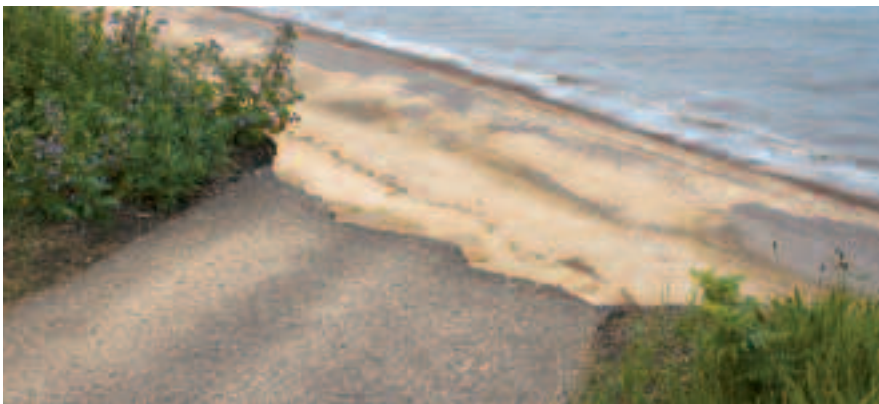
Erosion has brought this coastal road in Suffolk to an abrupt end 40ft above the beach
